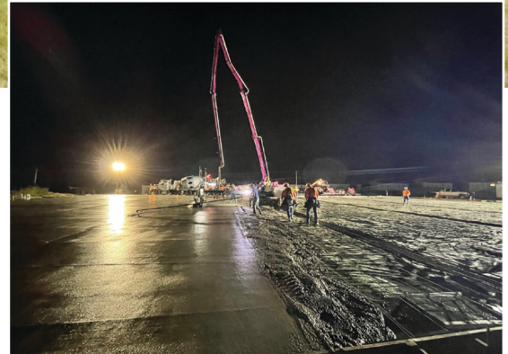
Early morning placement of the slab on grade to beat the heat for a better concrete finish.
