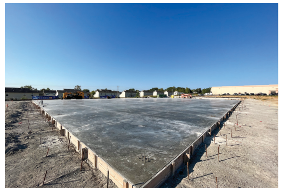
The finished slab on-grade, with curing compound, waiting for concrete strength before starting structural steel erection.
